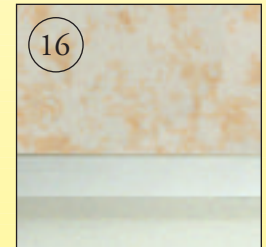
16 Bed cladding in Sealux-N on strip
